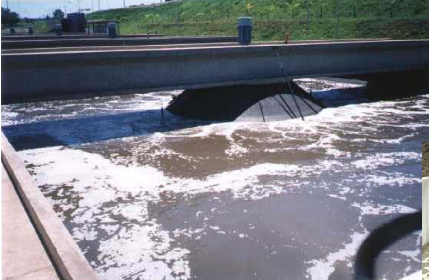
Surface Aerators in Aeration Tank
